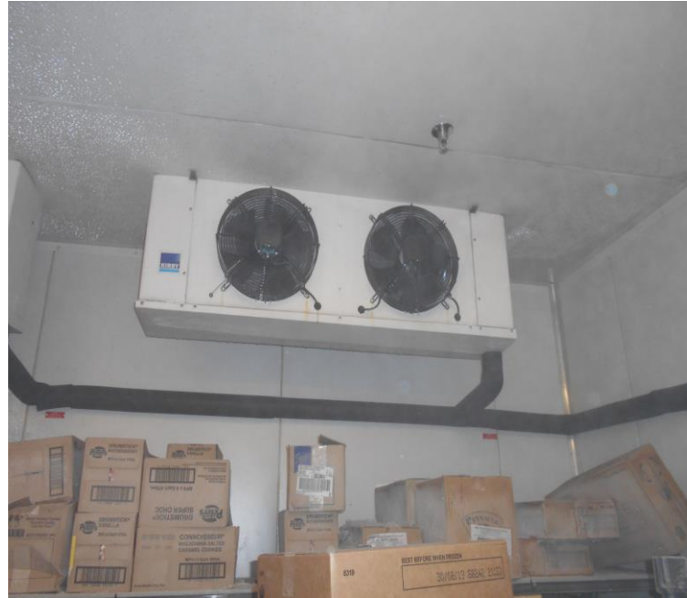
Post Installation LT Room – No Ice build up either Evaporator
