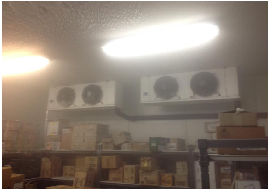
Pre Installation LT Room – Ice build up on Evaporators / fan motor blown
