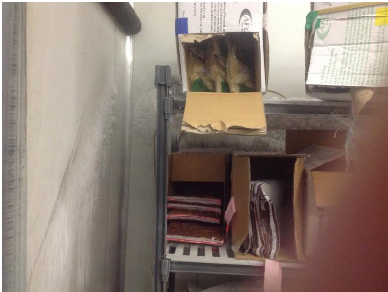
Pre Installation LT Room – Ice build up on Walls
