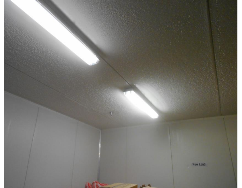
Post Installation LT Room – No Ice build up on Roof or Walls
