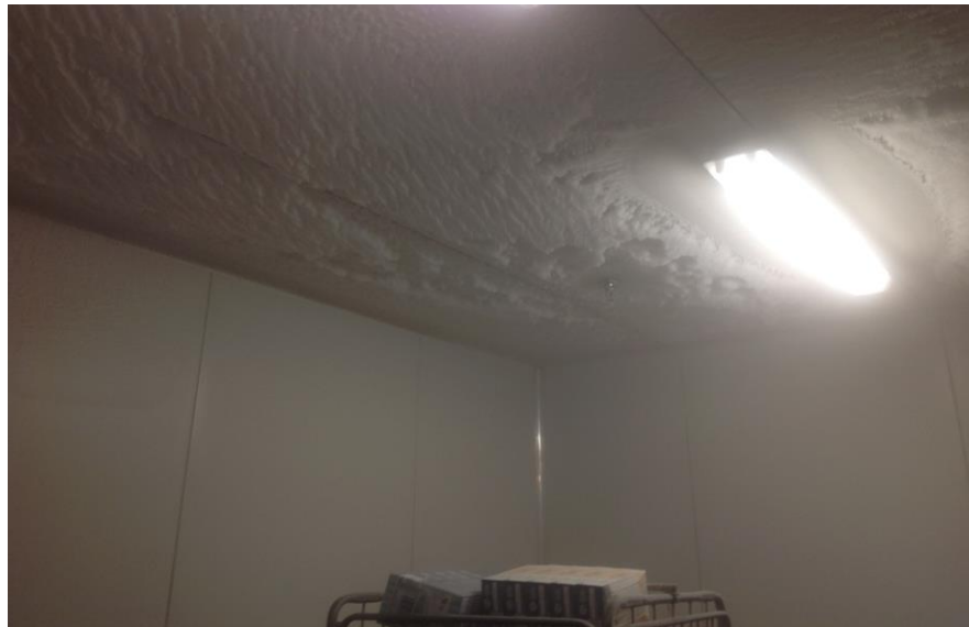
Pre Installation LT Room – Ice build up on Roof
